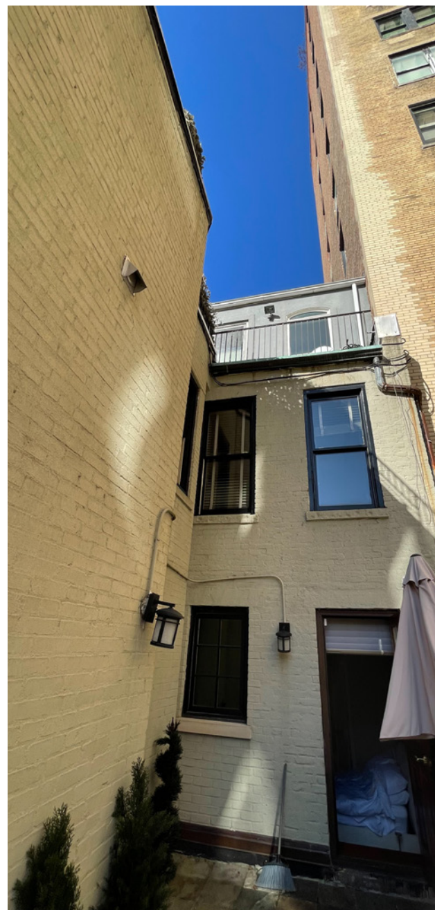
2. View on the roof of the two-story rear extension looking at the original rear
